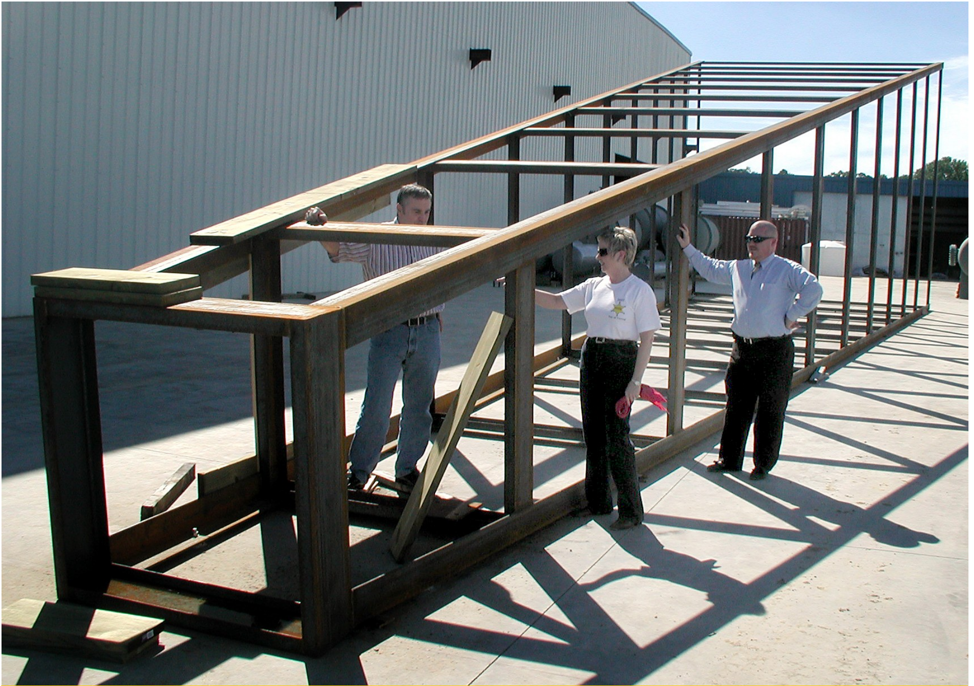
Project team members inspect a section of the new derrick's steel underframe.
