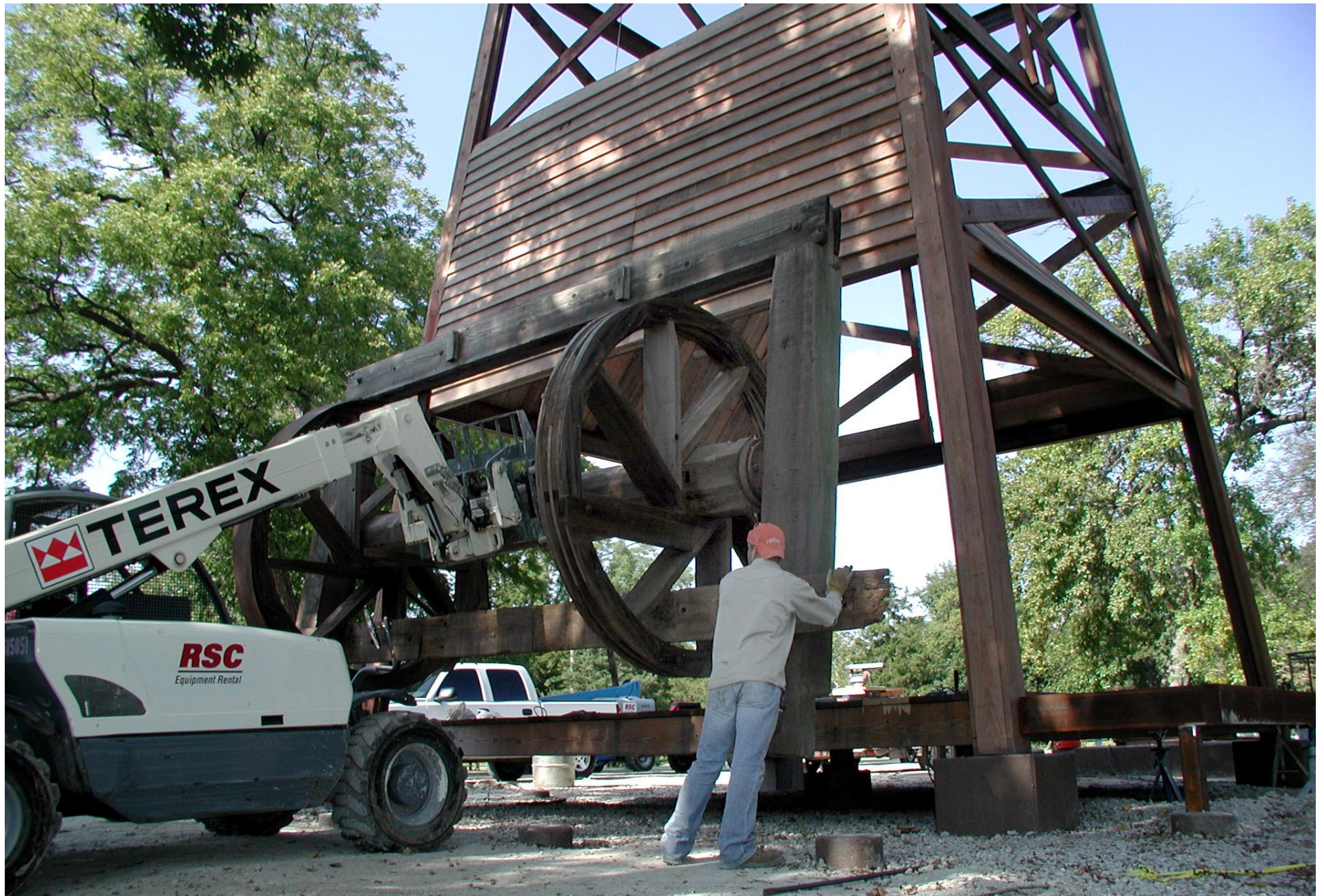
The “bull wheel” cable spool that was salvaged from previous rig reproduction and installed in the new derrick.
