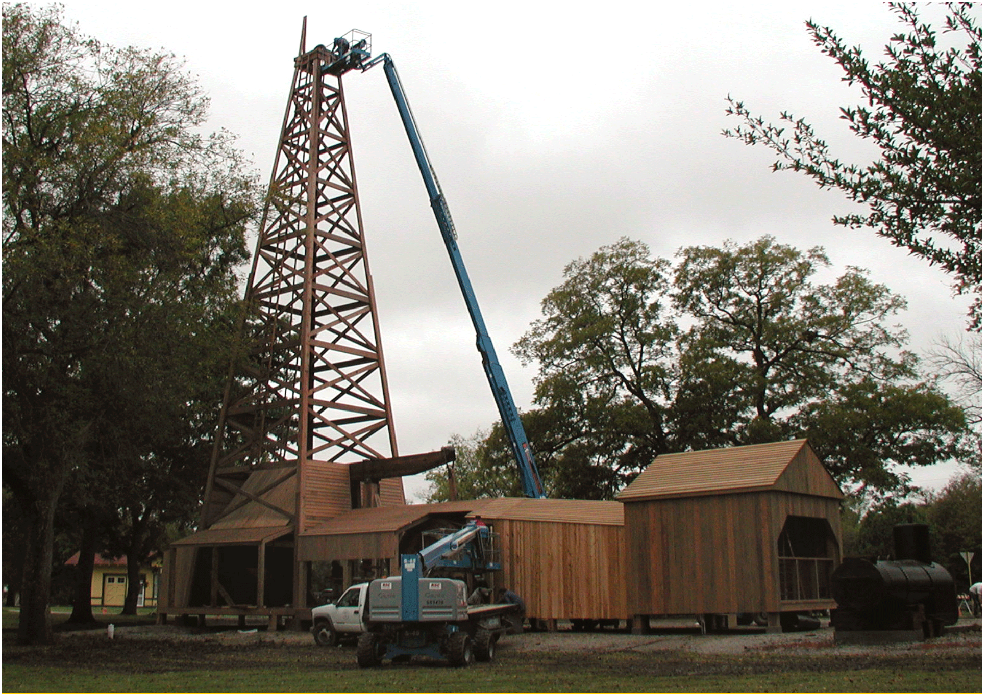
The derrick is “topped off” with the installation of a large pulley in the rig crown.
