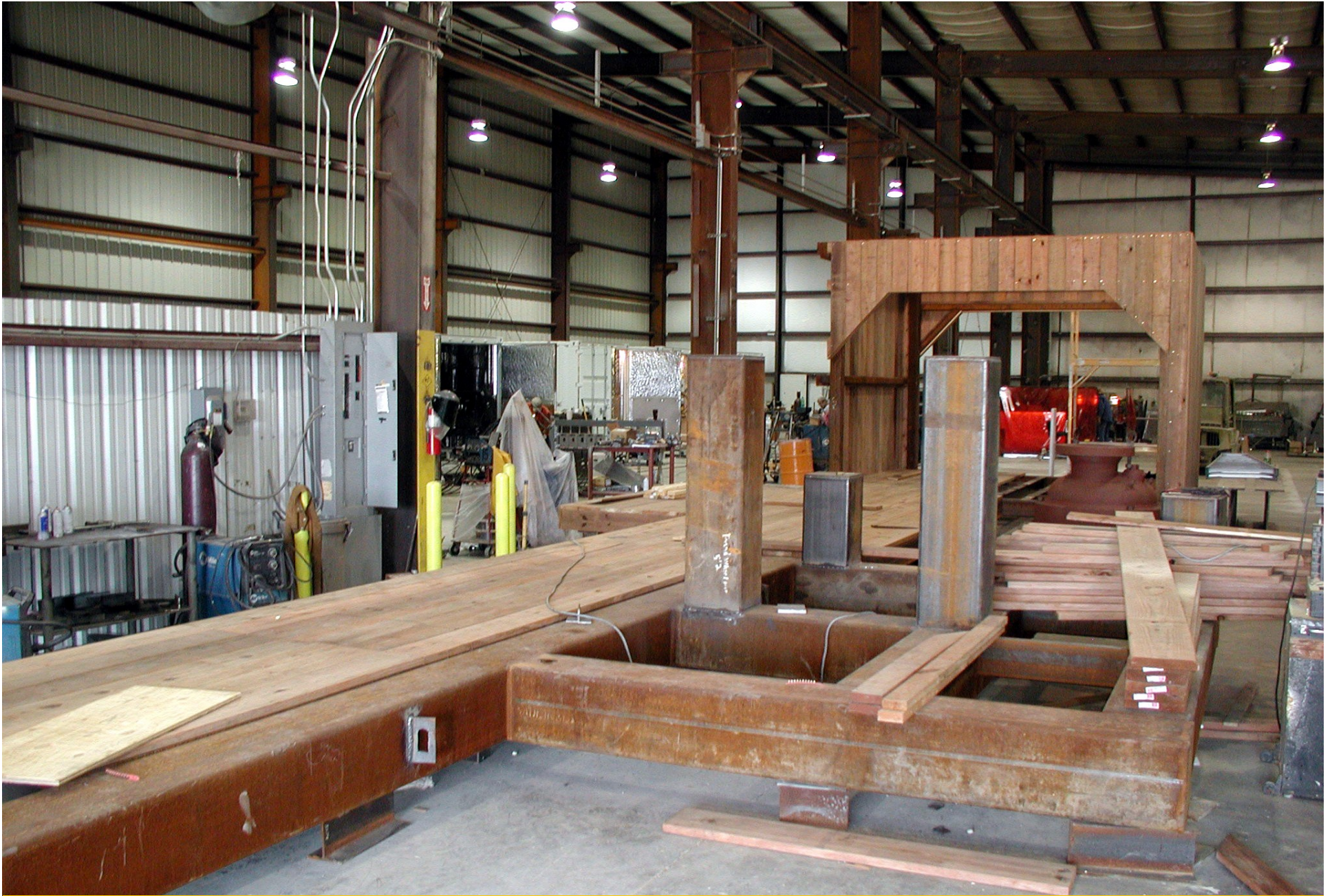
The derrick deck and engine house are constructed with steel frames at the indoor shop of SMC, a Bartlesville firm that built the derrick.
