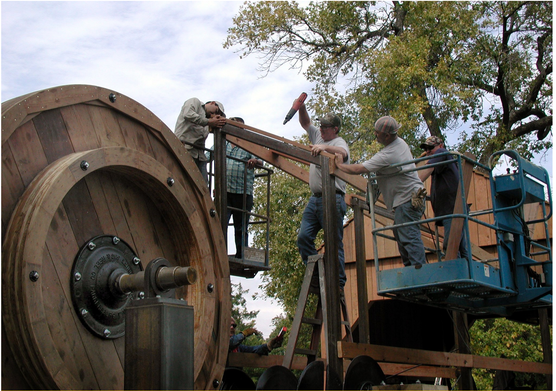
The huge wooden band wheel was built from scratch using original iron fittings.
